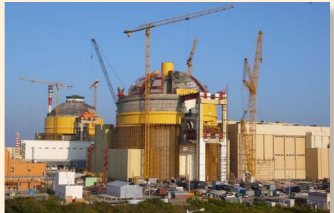
Kudankulam nuclear power plant, India
