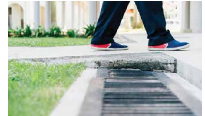
Concrete slabs have also been placed over drains, making it safer for elderly pedestrians.
